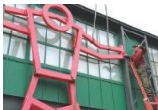
Kelley Welding Inc.'s shop foreman with Kelley Welding, works to position one of the figure's arms.
